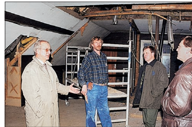
Taket i Logesalen falt ned.
